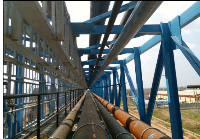
Station Piping Package for NTPC Solapur Super Thermal Power Project (2X660 MW)
