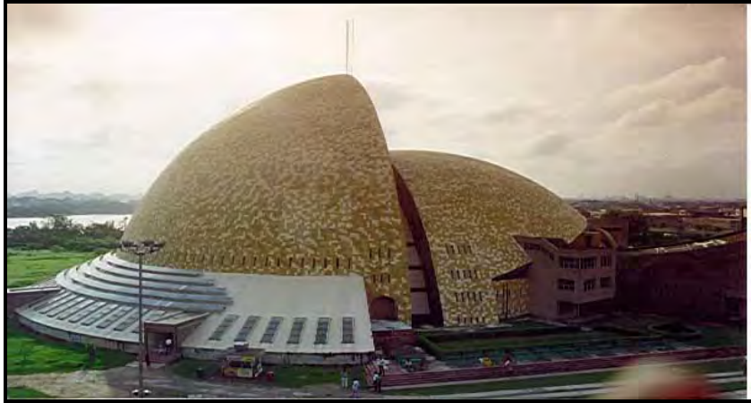
Construction of Convention Centre Complex Building including Piling Work at Science City for National Council of Science Museums at Kolkata (Height of Dome – 42 m)
