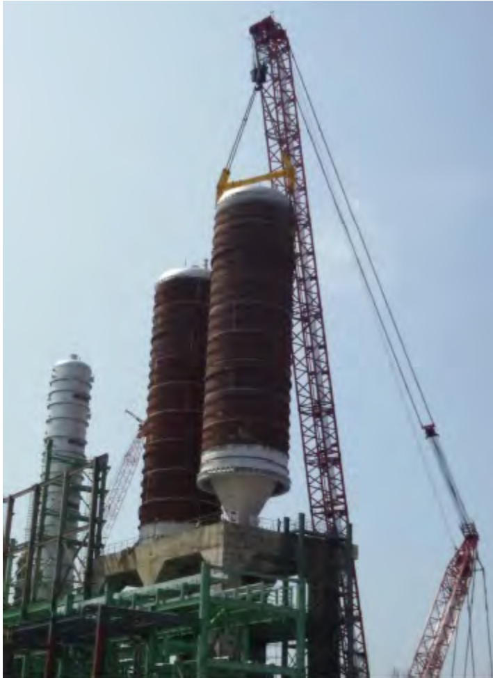
Erection of Two Coke Drums of 575 MT at DCU, CPCL, Chennai Site by Main crane 1250 MT capacity and tailing crane 550 MT
