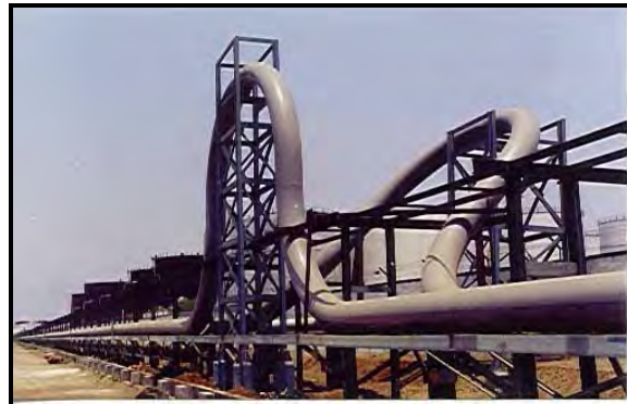
Cross-Country Pipeline for transportation of Black & White Oil for Oil Terminal of Indian Oiltanking Ltd.
