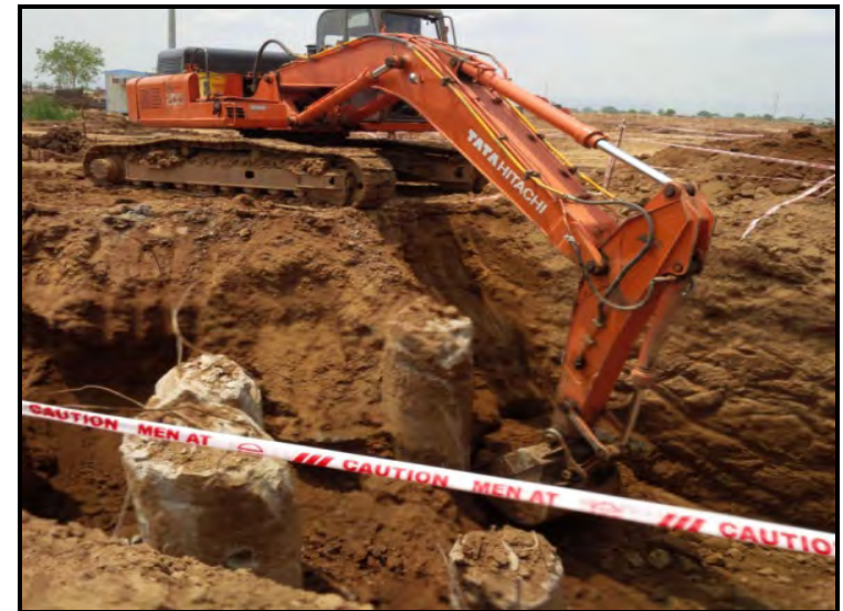
Area Grading and Construction of in plant Roads for 2 X 800 MW Unit at Gadarwara STPP of NTPC
