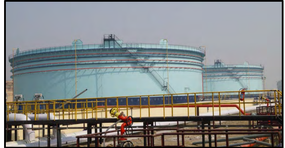
Steel Storage Tanks at Kanpur Terminal of HPCL
