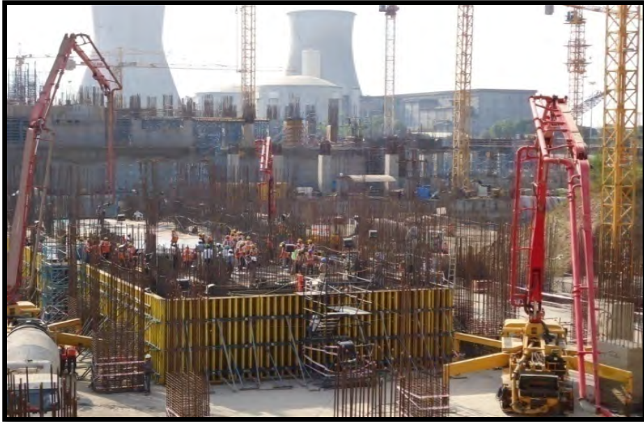
Civil & Structural Steel Work for Balance of Turbine Island Package for 2 X 700 MW Kakrapar Atomic Power Project (Unit 3&4) of Nuclear Power Corpn. of India Ltd. for Dodsai Enterprises Pvt. Ltd.
