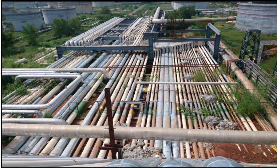
Offsite Piping at Mangalore Refinery & Petrochemicals Ltd.
