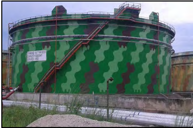
Storage Tanks at Numaligarh Refinery Ltd., Siliguri
