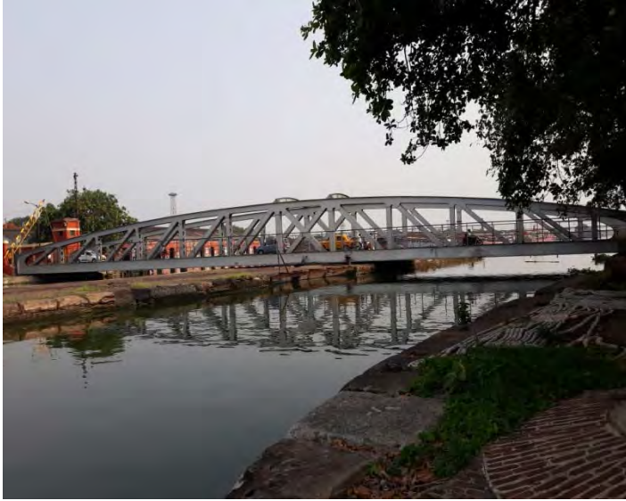
Repair of Swing Bridge at Kolkata Dock System for Kolkata Port Trust
