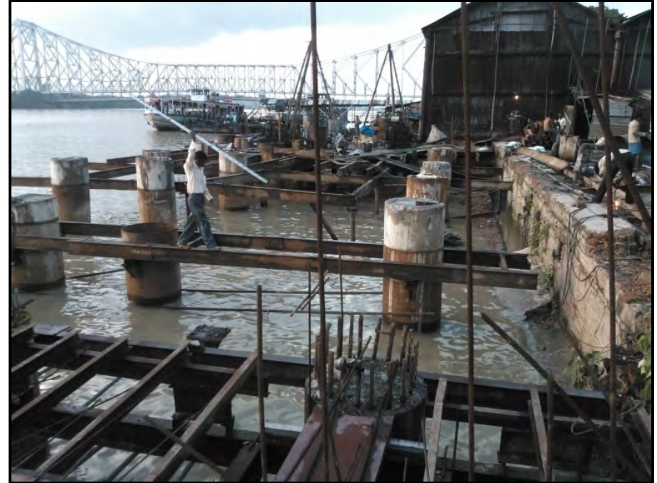
Construction of RCC Deck Slab supported on RCC MS lined Bored Pile of 1000mm dia., beam including pavement for Hooghly River Front Development Work of Kolkata Municipal Corporation
