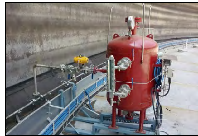
Automatic Rim Seal Fire Protection System for External Floating Roof Tanks for IOCL, BPCL & HPCL at various locations
