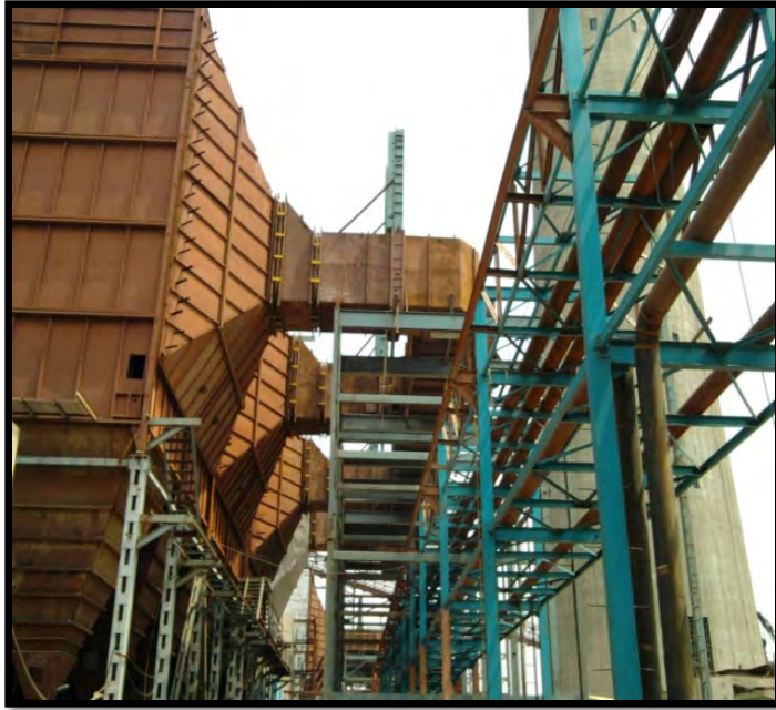
ESP, Boiler & its Auxiliaries, etc, of 500 MW Unit-6 for NTPC Rihand Super Thermal Power Project 2X500 MW for BHEL
