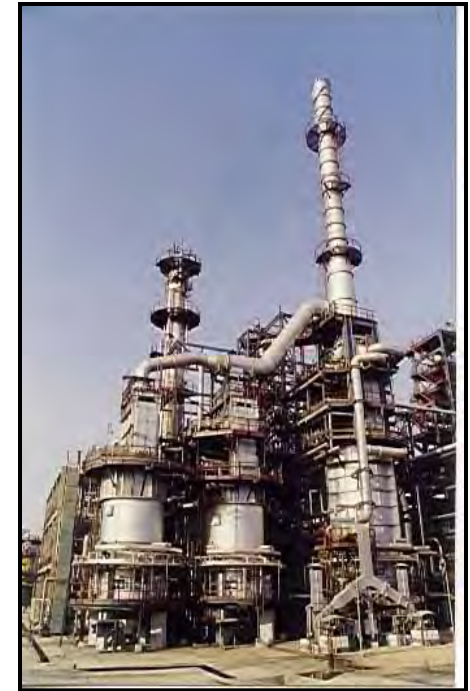
Turnkey Construction of 3 Nos. Non-IFP Heater in Panipat Refinery Project of IOCL , for Hydrotreater Reactor, Reboiler & Stabilizer Reboiler
