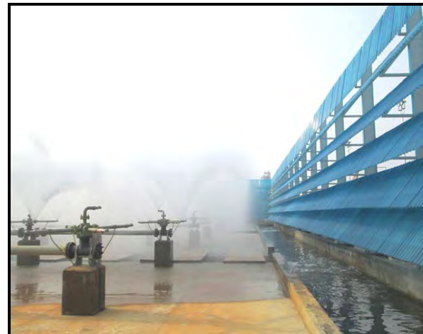
3000 m 3 /hr Mist Cooling Water System for Gas Cracker Unit on Turnkey Basis at GAIL Pata
