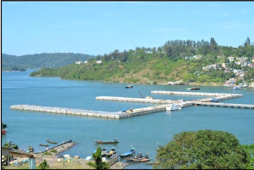
Construction of RCC Finger Jetty with Approach at Junglight in Port Blair for Andaman Harbour Works
