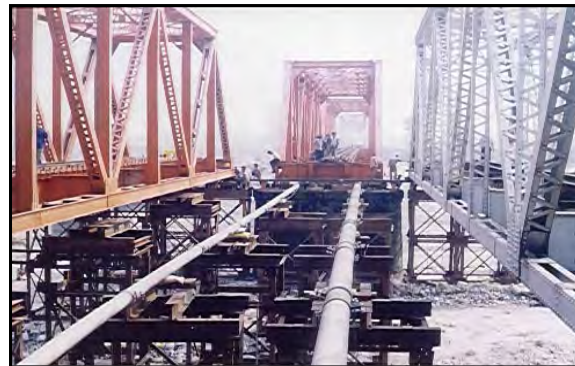
Regirdering of 7 spans X 45.70 metre each of Diana Bridge for Northeast Frontier Railway
