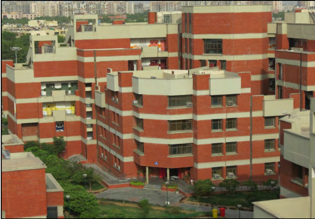
Construction of Administrative Block (G+3), Library Block (G+2) and 5 Nos. Academic Block (G+6) at Guru Gobind Singh Indraprastha University, Delhi.
