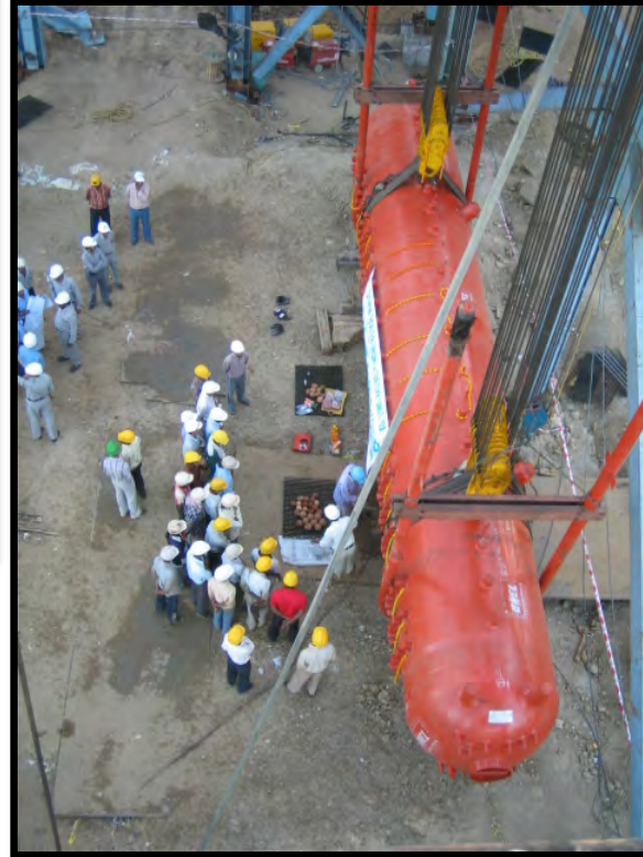
Boiler, Air Pre-Heater & Piping of 2 x 210 MW, Unit - 4 & 5, Bakreswar of West Bengal Power Development Corpn. Ltd.
