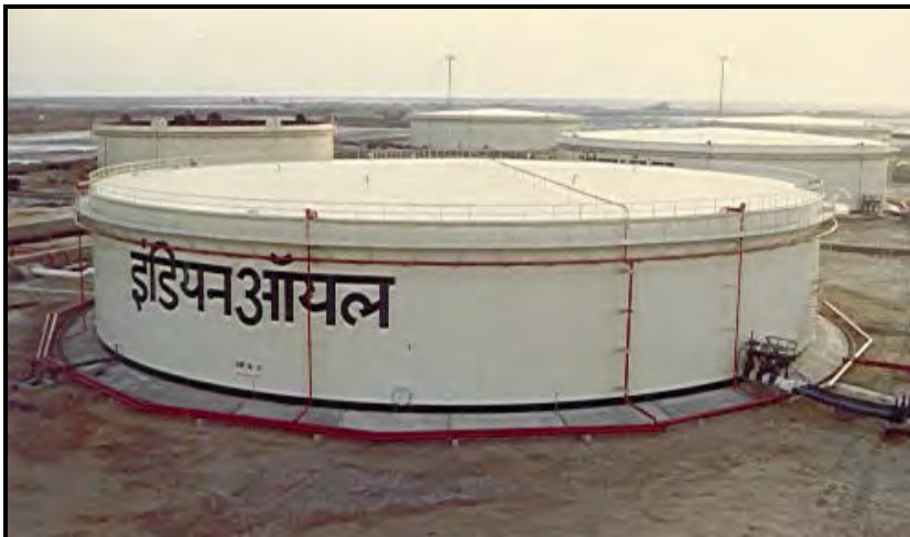
Product Storage Tanks with connecting pipeline at IOCL Panipat
