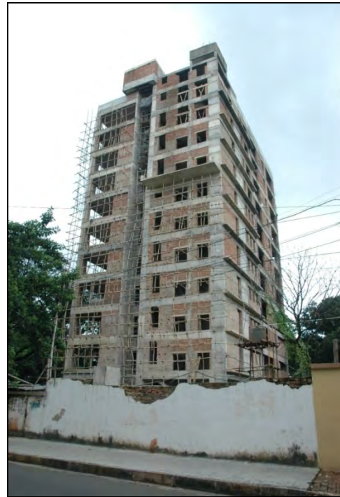
Construction of B+G+10 Storied Residential cum Office Building at Kolkata for Visa International Ltd.
