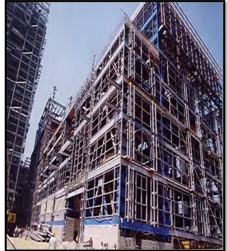
Power House Building 2X500 MW Simhadri Thermal Power Station of NTPC
