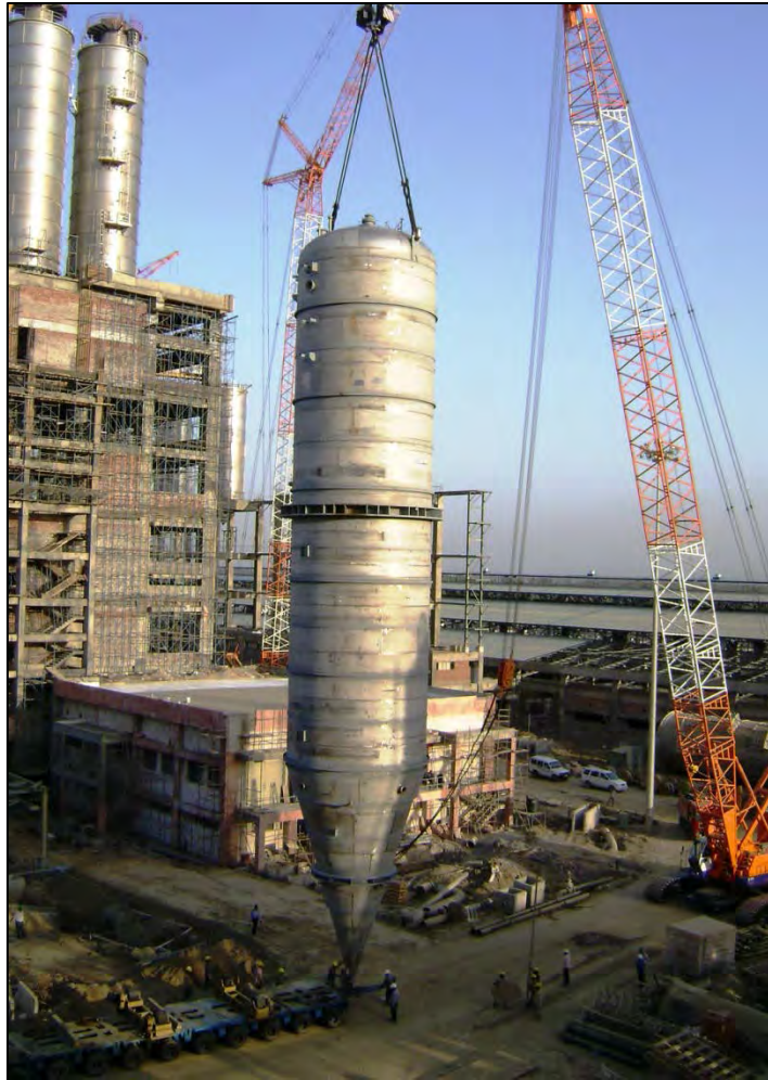
RA Stripper ( 6.40 Mtr Dia 35.20 Mtr Long 75 MT weight ) being erected at LLDPE unit of IOCL, Panipat with 450 MT Crane and 250 MT Trailing Crane
